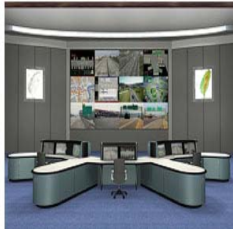
Traffic Management Center
